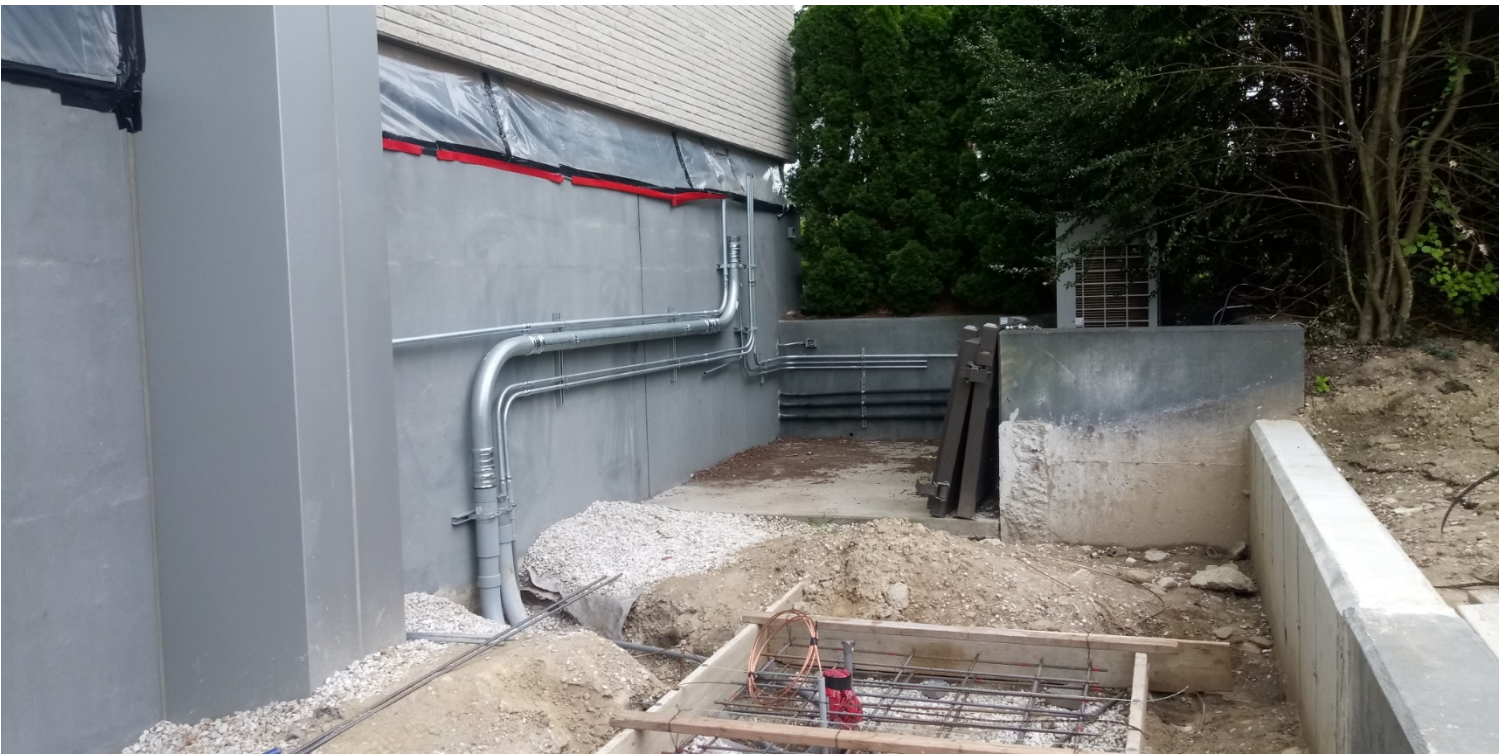
Mechanical Pen – PVC conduit & fiber routing from Jefferson St. / Generator pad reinforcing.
